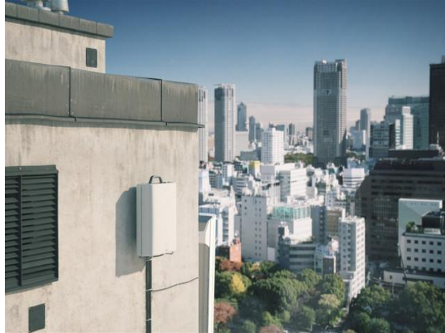
BTS Radio Distribuida 1 Sector Wall
