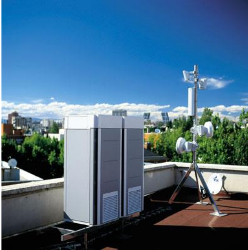
GSM Site Outdoor RoofTop
